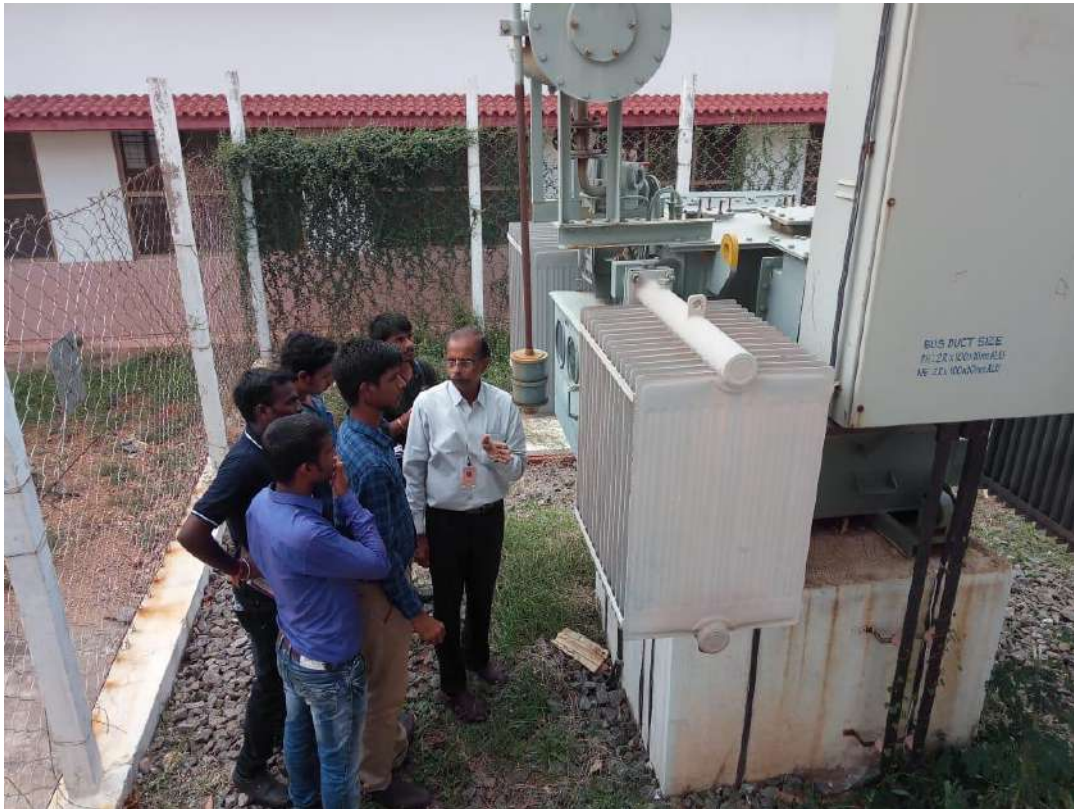
Dr.Kalyankumar, Professor/EEE explaining the operation of transformer in substation
